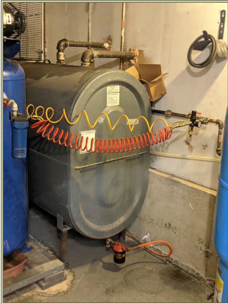
275-gallon #2 fuel oil above ground storage tank near back of fire station building
