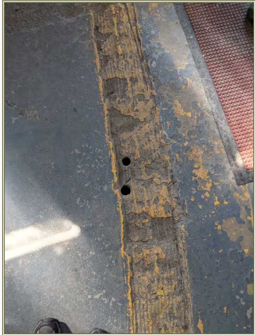
Holes drilled through the concrete floor to assist with drainage issues
