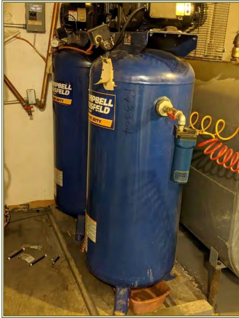
Two compressors next to oil tank
