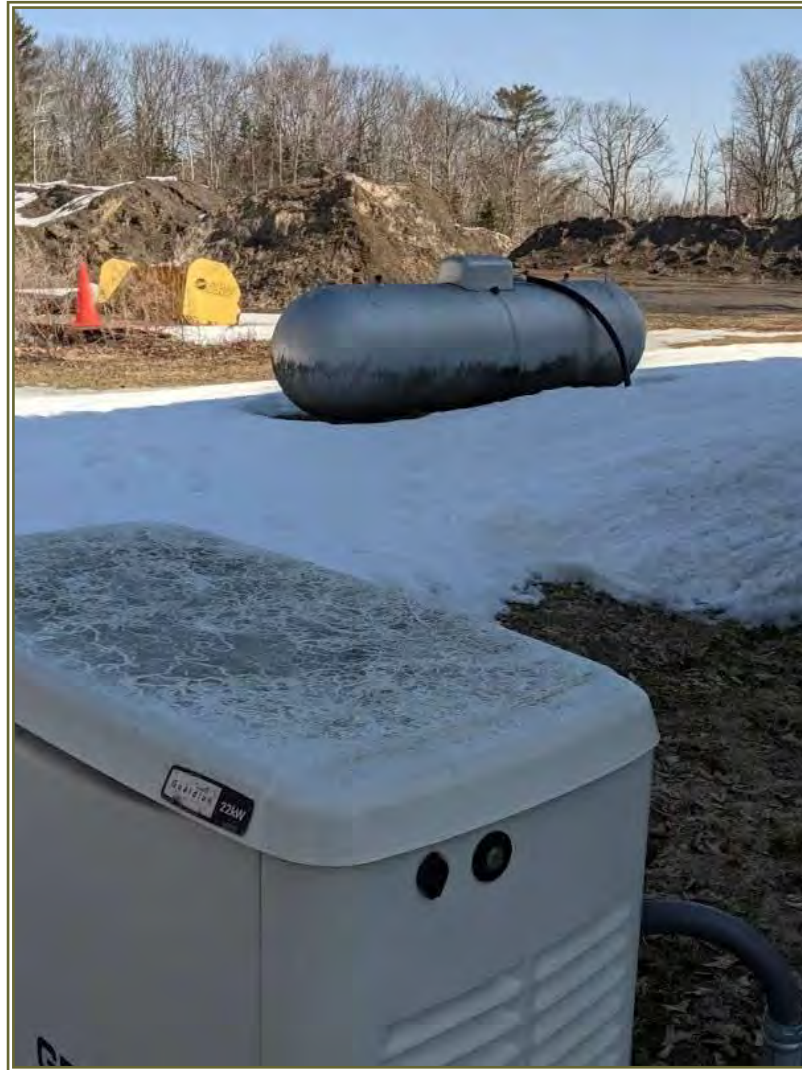
Generator and propane tank near northwest corner of Fire Station Building looking northeast
