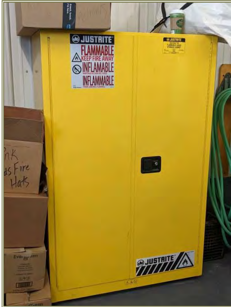
Flammable cabinet in the newer western portion of the Fire Station
