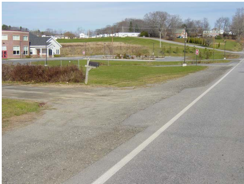
Figure 6. Sidewalk on Rt. 141 ends at Robbins Rd. instead of at the East Side school or Keene Mobile Home Park
